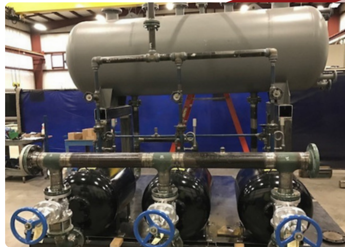
Condensate Receiving Skid
