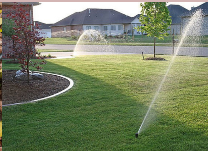
Water coverage assessments allow for optimized efficiency
