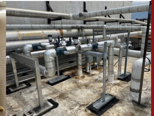
Roof Top Ammonia Valve Station
