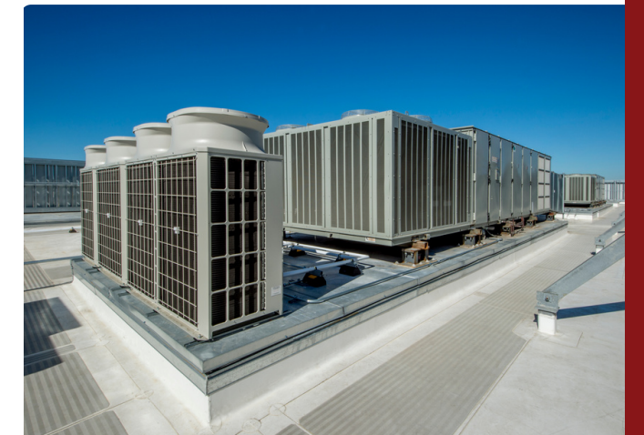
From residential units to large commercial units, we service all makes and models
