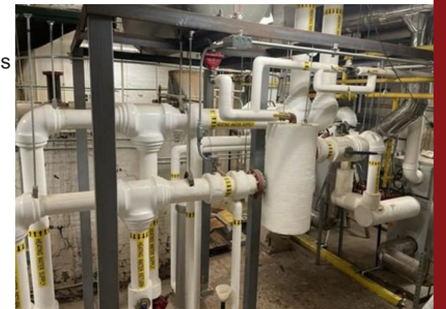
Hydronic Heating System within Mechanical Room
