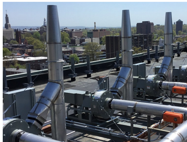
Roof Top Exhaust Air Units
