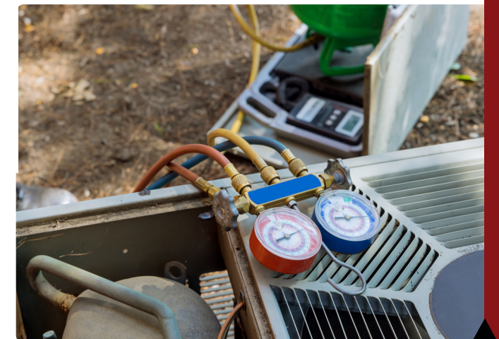
We perform seasonal tune-ups to keep your HVAC equipment running smoothly
