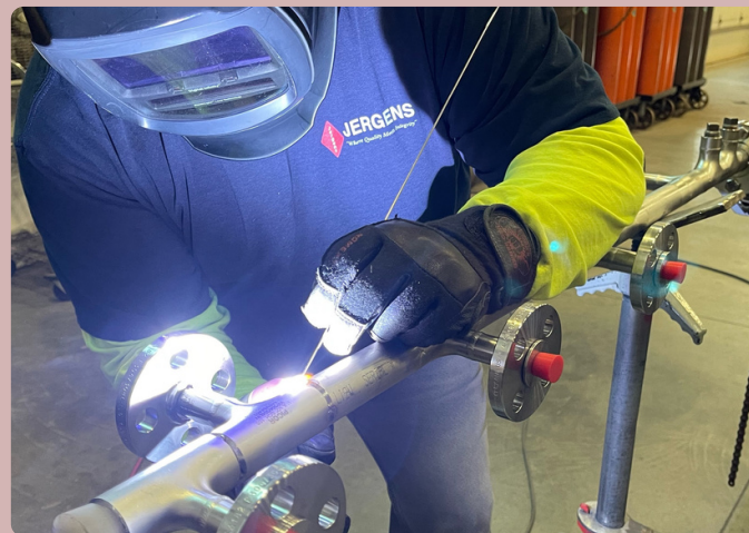
Small-bore, stainless steel, pharmaceutical process piping
