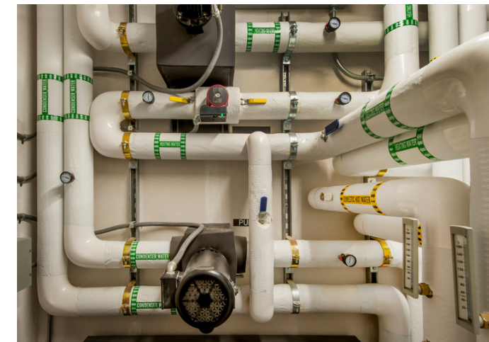
Chilled Water System
