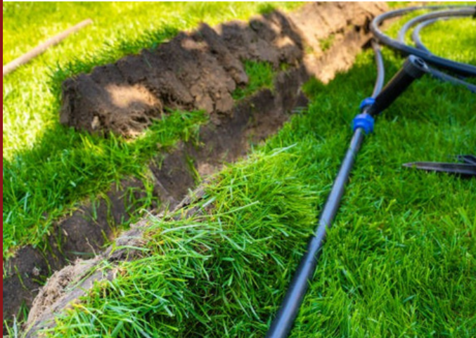
Fully designed layout done for new installations
