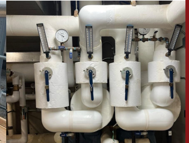
Steam Valve Station
